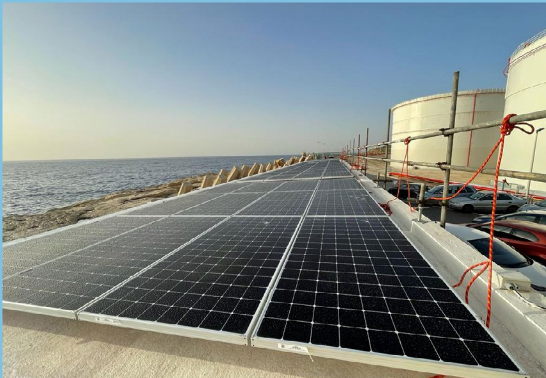
Solar panels installed at the Malta terminal in 2022.
